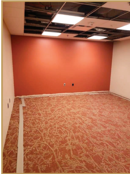
By late fall 2018, interior work in the newly expanded north annex was almost complete.
