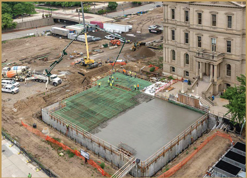
The roof of the new CUP was poured in the first half of August in 2018, marking a major project milestone.
