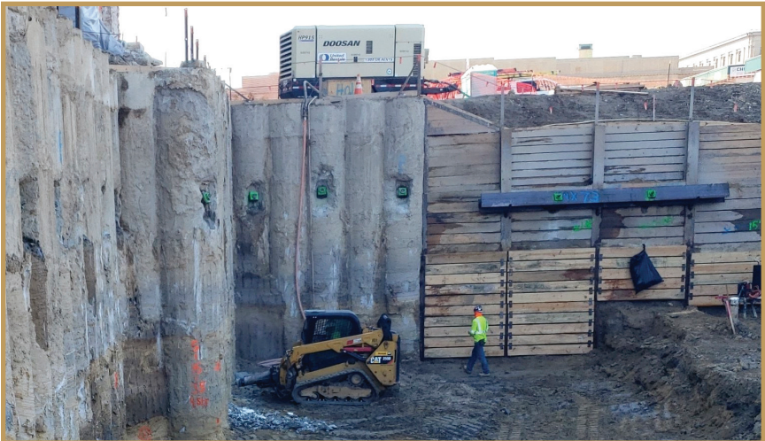
The excavation site was secured using a concrete secant wall (as seen on the left of this image) and soldier piles with wooden lagging (as seen on the right). Together these enforced the Capitol's foundation and held back the dirt.
