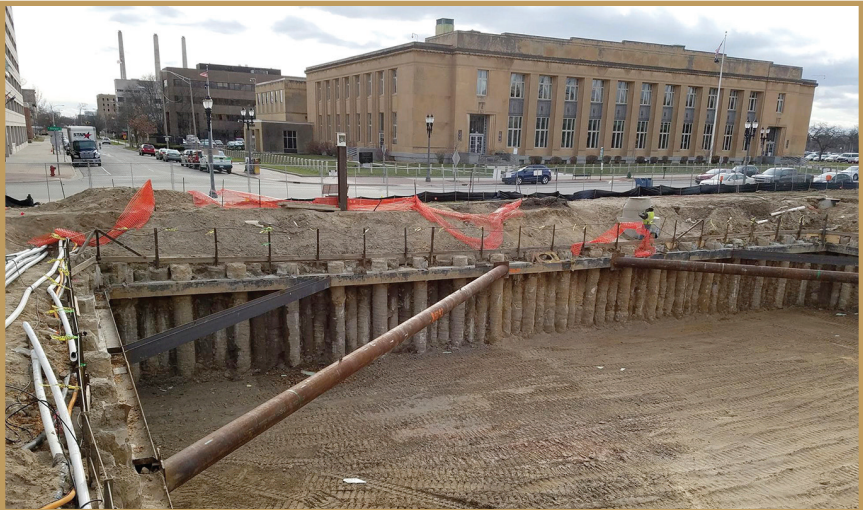
The piles (or posts) that comprised the ERS held back the earth around the construction site, preventing erosion.
