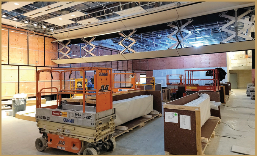
The silver framework that forms the center of the Skyfold partition looks like a giant metal pantograph.
