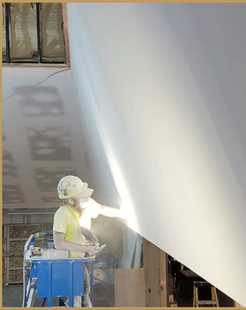
A workman examines a layer of Acoustibilt finish on an angled wall beneath a skylight.
