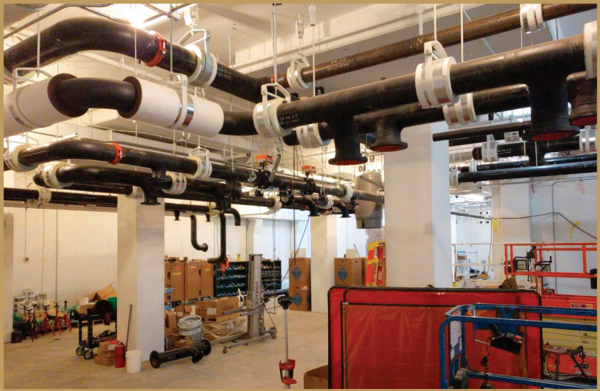
The CUP is full of overhead piping that comprises part of the geothermal system.
