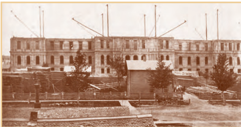
The State Capitol under construction in 1875. Derricks rise above the walls, which have been completed to the second story.
